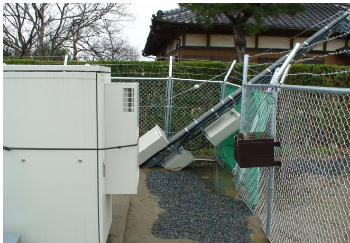
(a) Collapse of drawing pillar at NTT DoCoMo's base station
