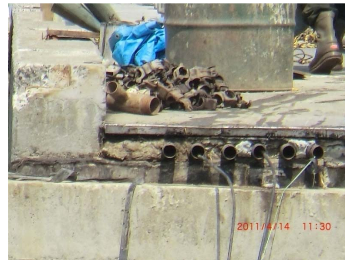
(b) Equipment damaged by falling bridge
