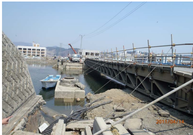
(a) NTT manhole exposed by destruction of riverbank protection
