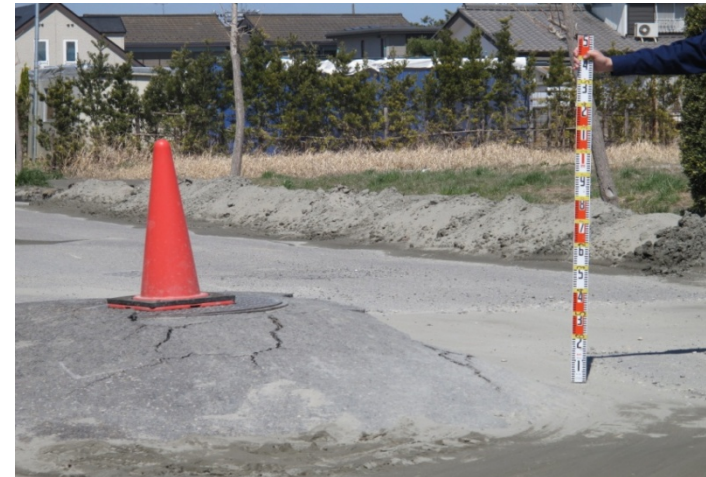
(b) Surfacing of NTT's manhole by liquefaction
