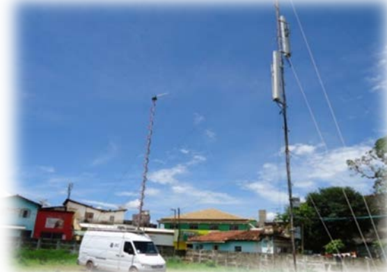
LTE Antenna and Mobile Unit
