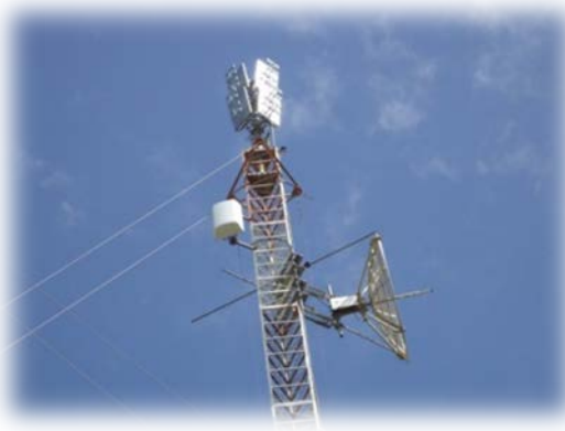
TV Transmitter Antenna
