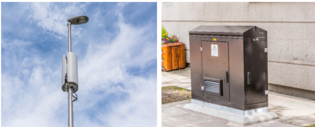
Figure 6: An example of a small cell antenna system and a street cabinet
