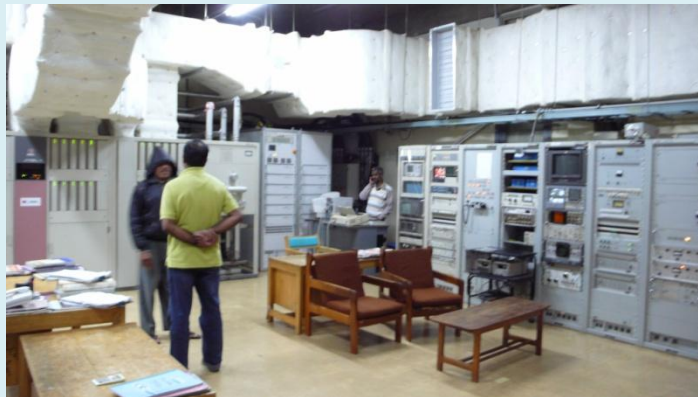
Figure 28: Equipment hall in SLRC broadcasting station at Piduruthalagala
