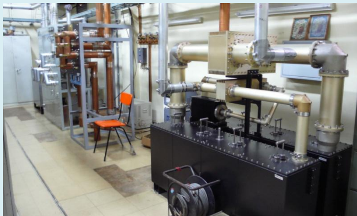
Figure 29: Band III combiner in SLRC broadcasting station at Piduruthalagala
