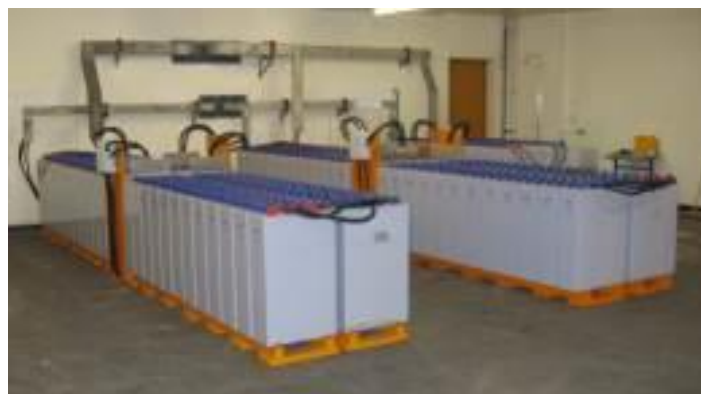
Figure I.1 – 48V multistring lead-acid battery in a telecom centre
