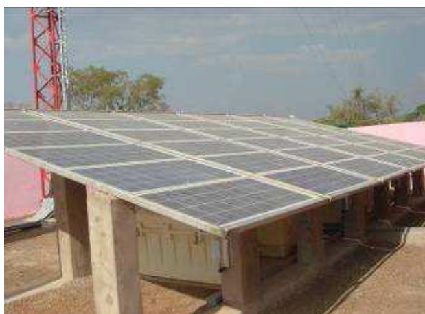
Figure I.6 – Example of a solar power system for a radio mobile base station equipped with ORYX® solar system equipped with Energys flooded tubular lead-acid battery referred to as OPZS (courtesy of Orange)
