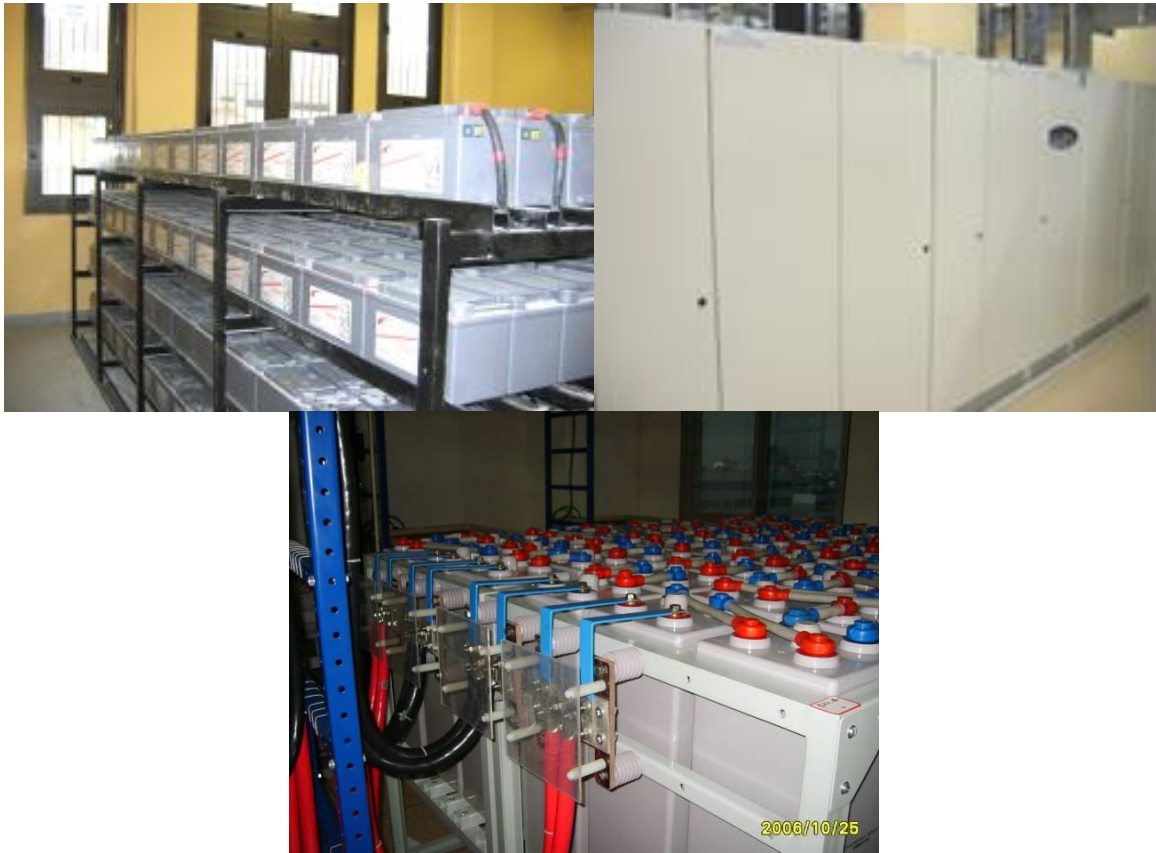
Figure I.3 – UPS multi-string batteries on shelves or in cabinets
