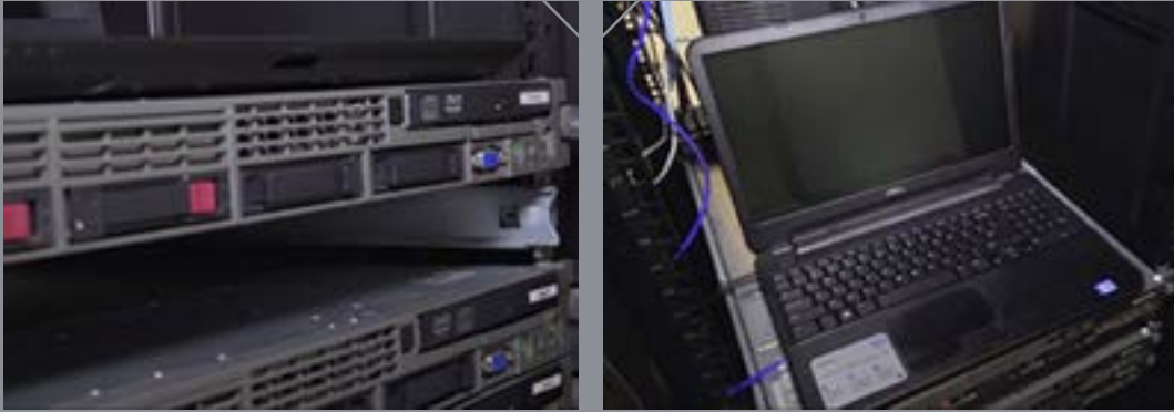
Servers of the established CIRT which are located at the premises of the Telecom Division
