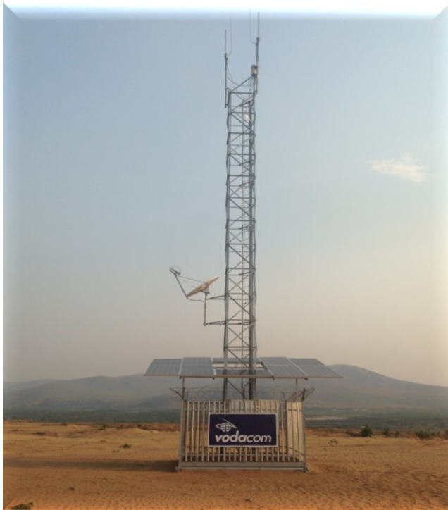
Solar based cell tower with GSM backhaul in DRC
