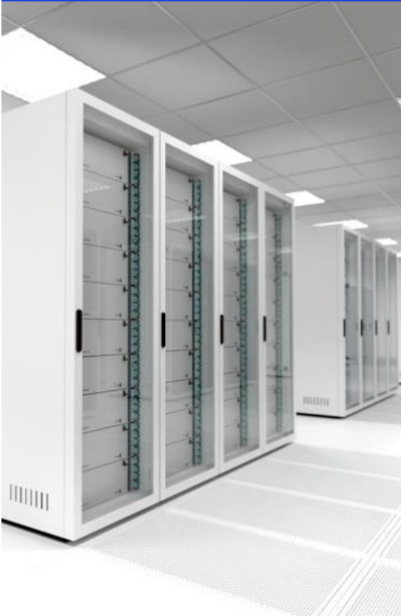
Inside the Data Center
