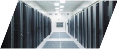
Compute, Network & Storage Pooled Resources Standardized Commercial Grade Solutions
