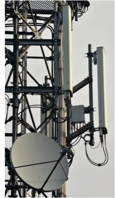
Satellite backhauling mobile stations in rural areas
