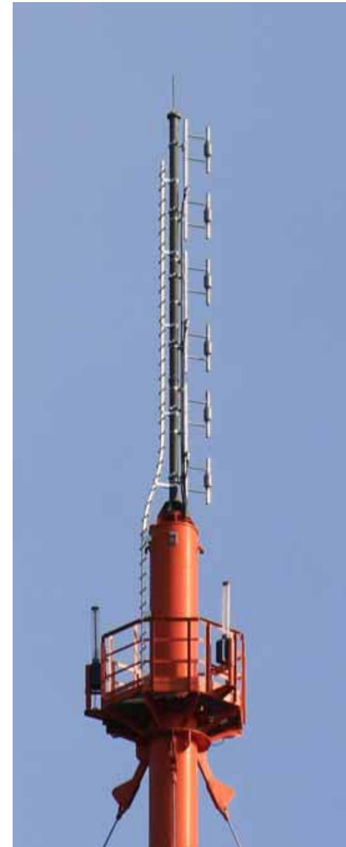
VHF Transmitting Antenna „Raichberg“
