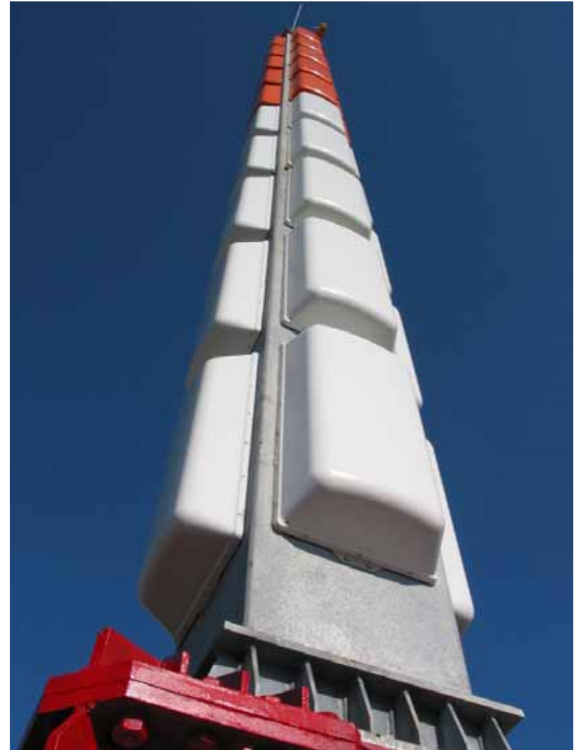
UHF transmission antenna
