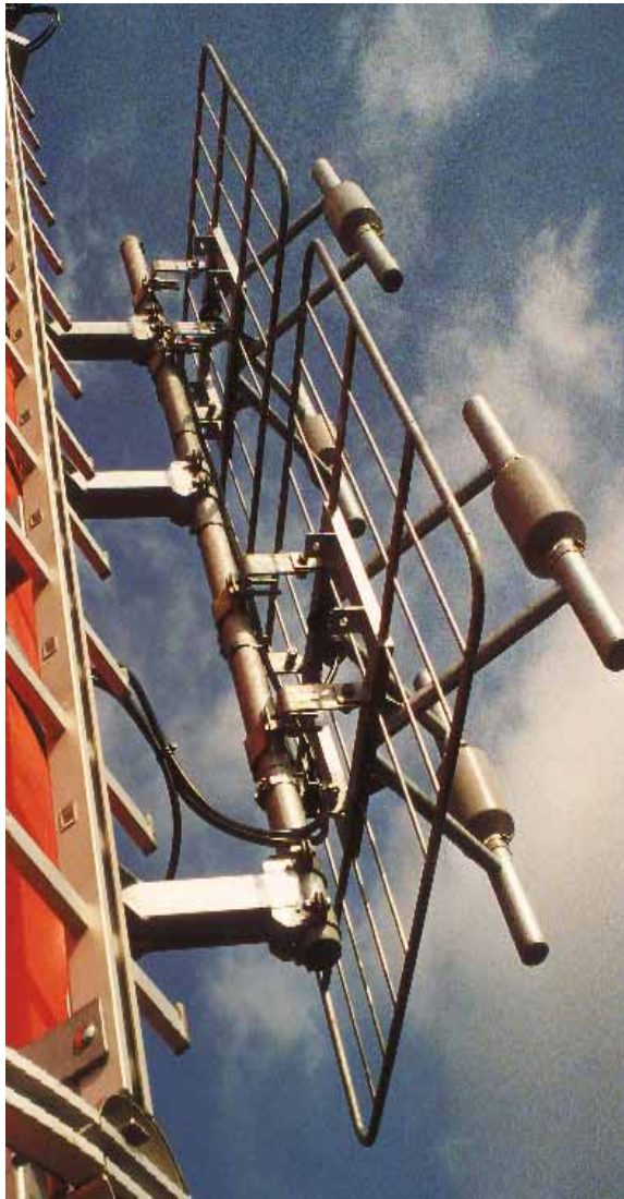
Panel Fixation Steelwork
