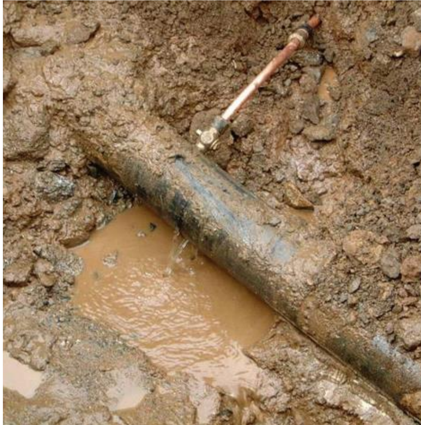
Underground leak running at low pressure (Brothers K , 2002)
