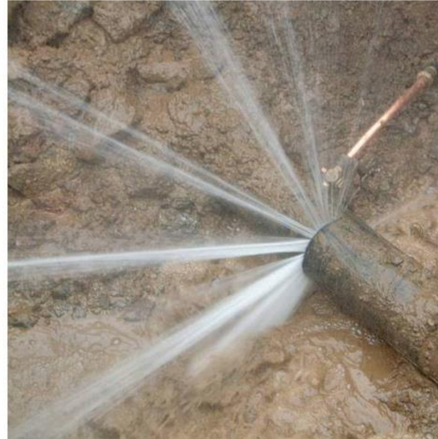
Underground leak running at high pressure (Brothers K , 2002)
