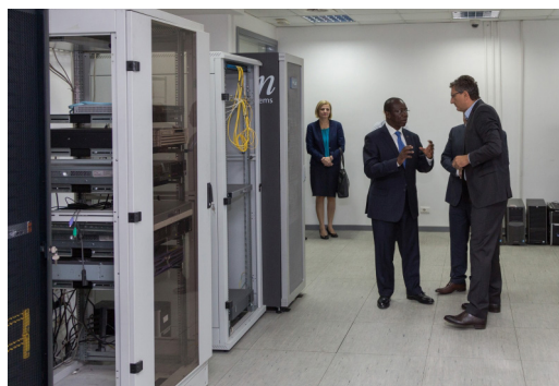
IXP center in Montenegro
