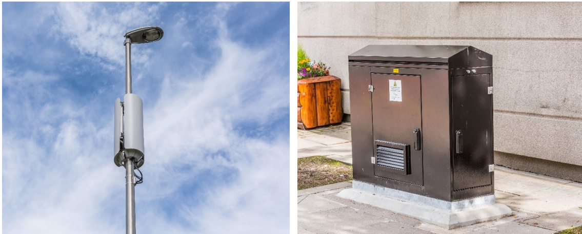
Figure 6: An example of a small cell antenna system and a street cabinet. Source: Wireless Infrastructure Group, 2018
