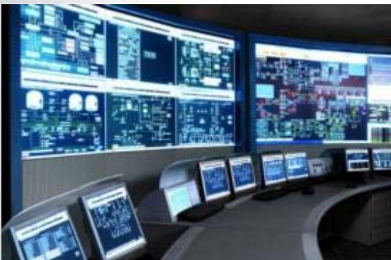
Control room in 60s, 80s and 2000s
