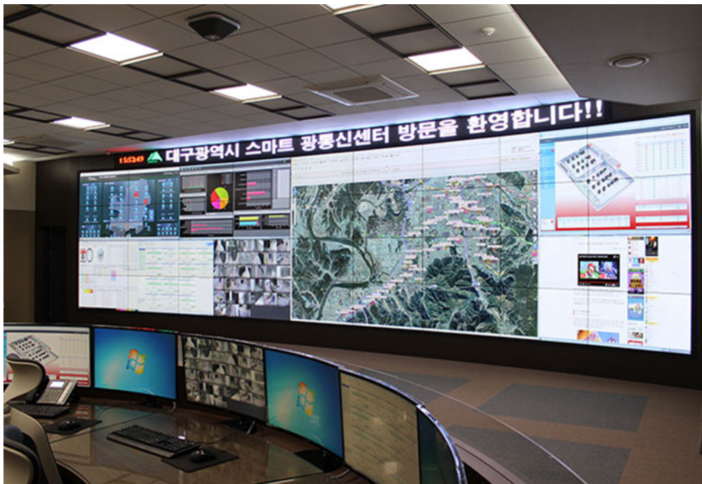
Figure 12: Daegu smart optical telecommunication centre
