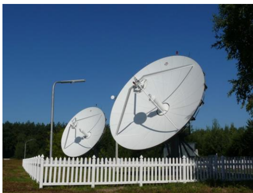
UCRF satellite monitoring station antenna system
