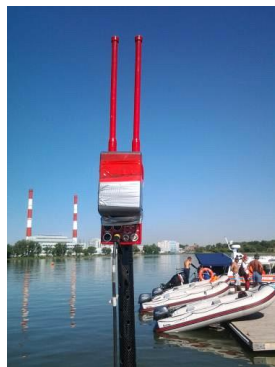
Wireless access station in Rowing Sports Center
