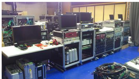
FIGURE 13 Line and transmission equipment
