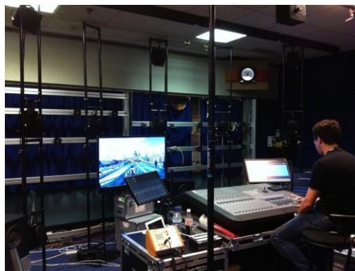
FIGURE 17 Main mixing room
