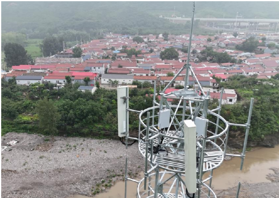
FIGURE 64 5G NR base station
