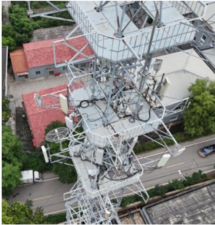
FIGURE 65 5G NR base station
