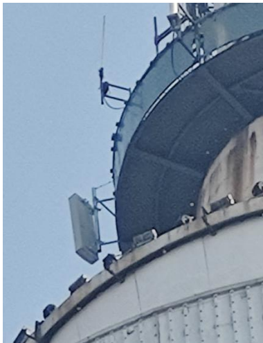
FIGURE 72 The location of the base station on the tower
