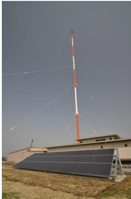
FIGURE A1-3 12 kW solar power generating facility
