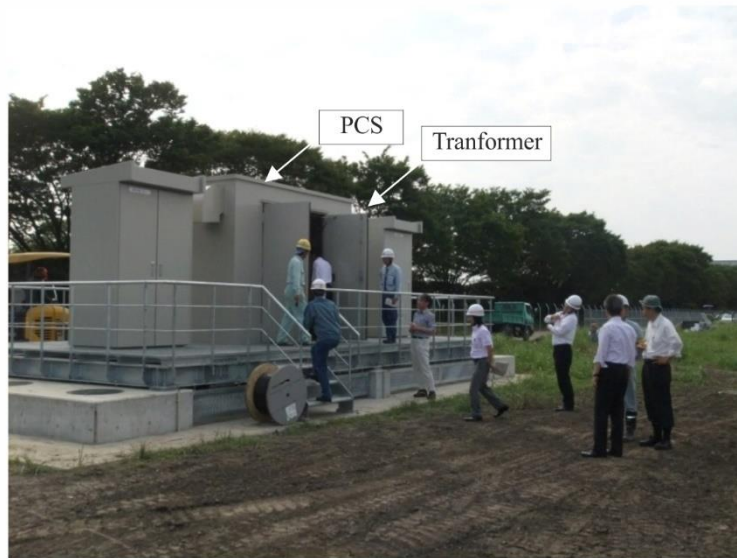
FIGURE 11 External power panels
