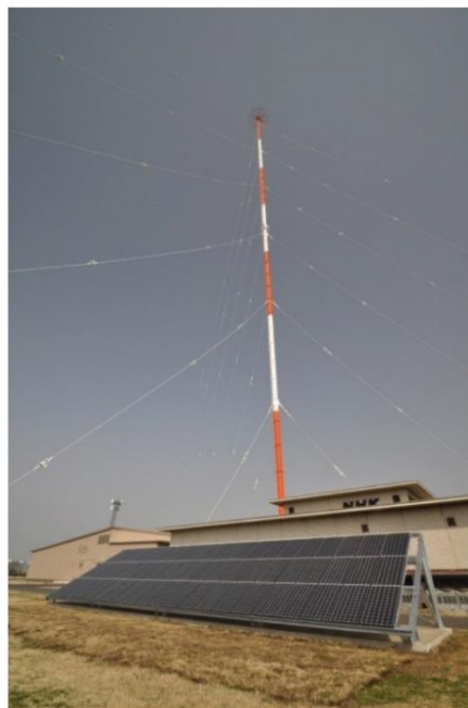
FIGURE 3 12 kW solar power generating facility
