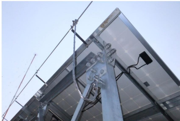
FIGURE 9 Lightning protection equipment
