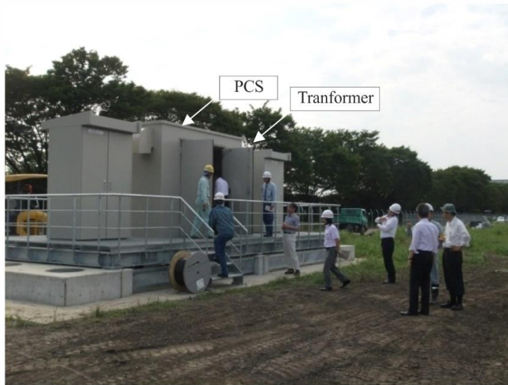
FIGURE 11 External power panels
