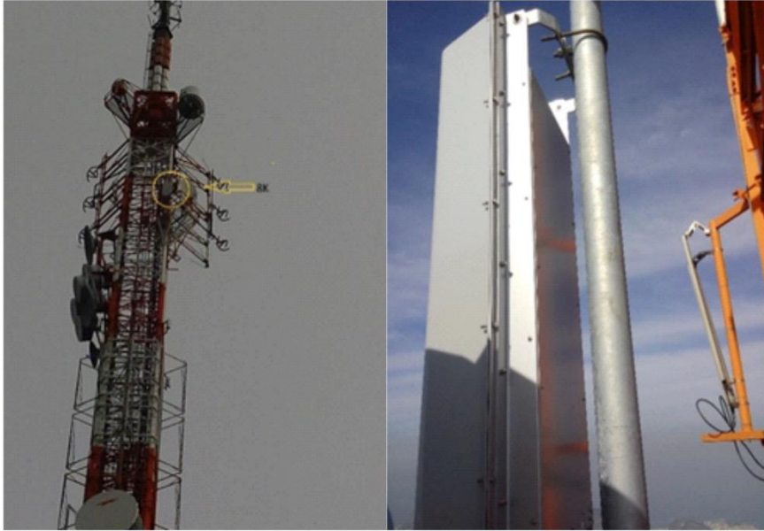
Transmission station antenna
