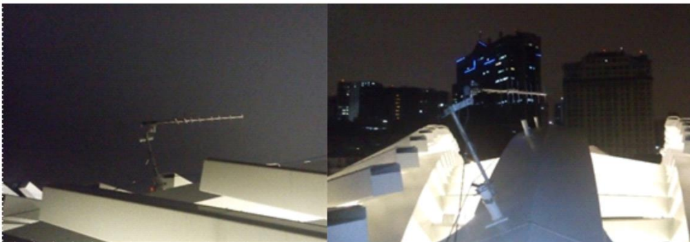
Reception station antenna
