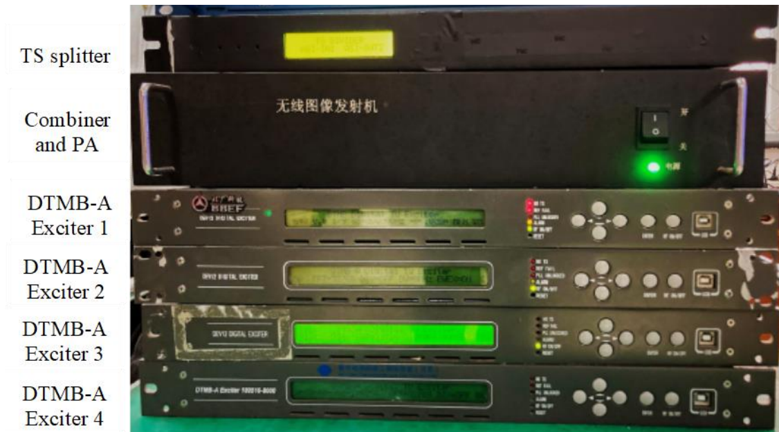
Equipment of transmitter site
