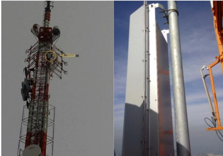
Transmission station antenna
