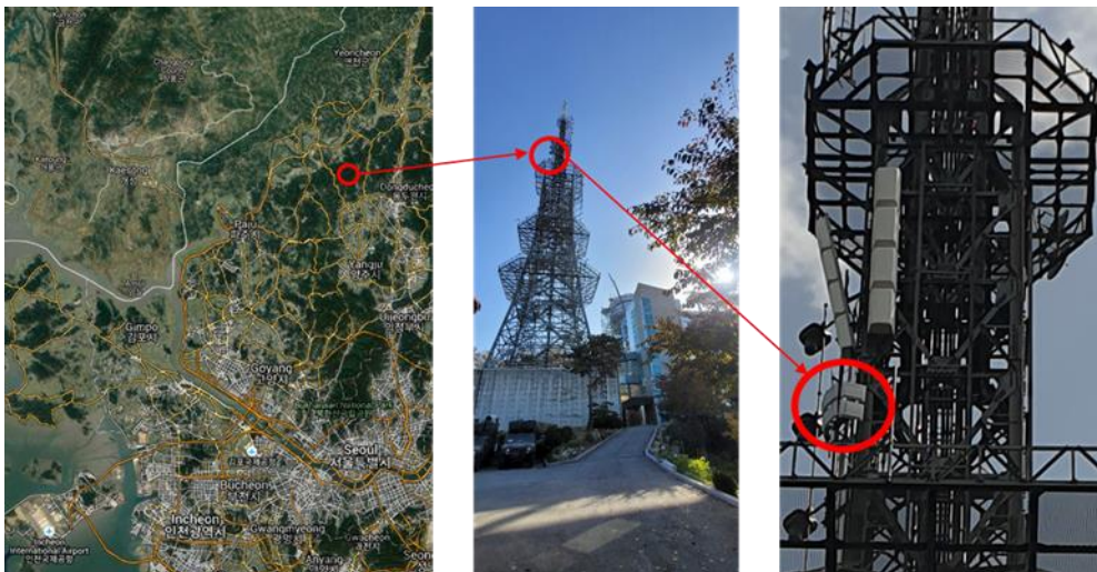
ATSC 3.0 MIMO transmission tower
