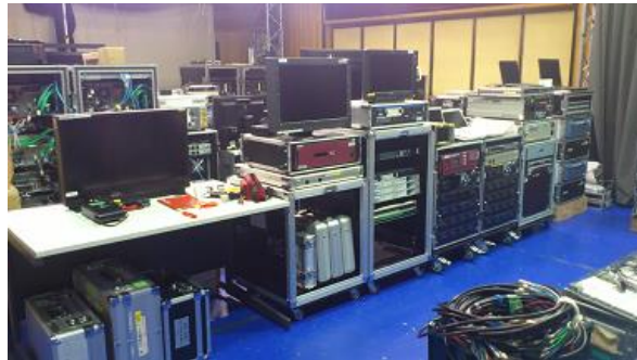
FIGURE 61 Line and transmission equipment
