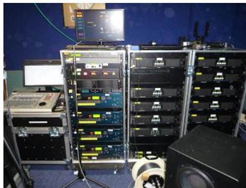
FIGURE 66 Sound equipment in the preview room
