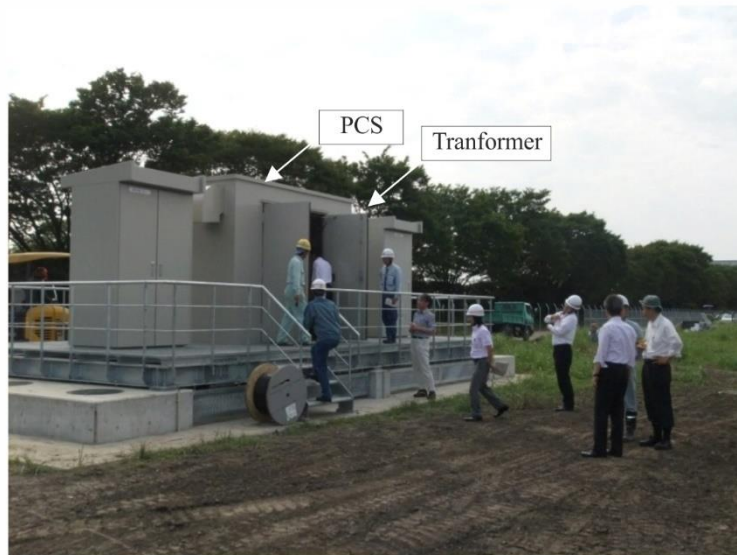
FIGURE 11 External power panels
