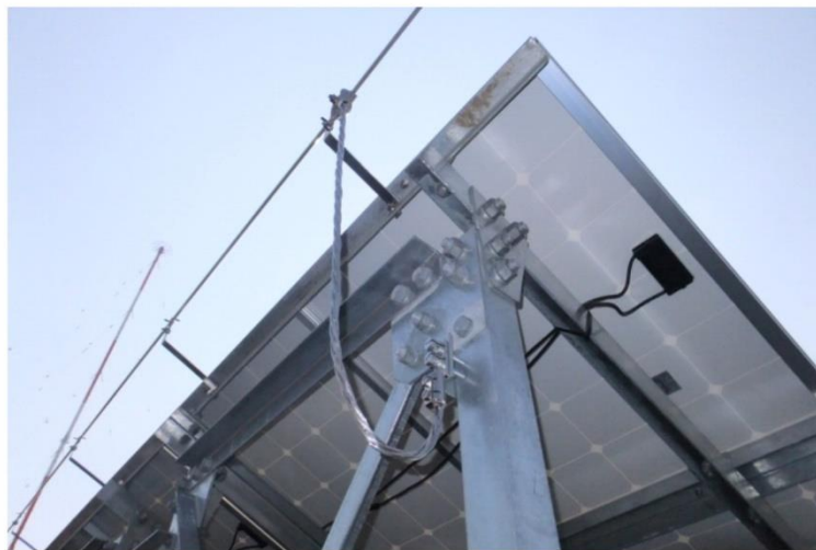
FIGURE 9 Lightning protection equipment
