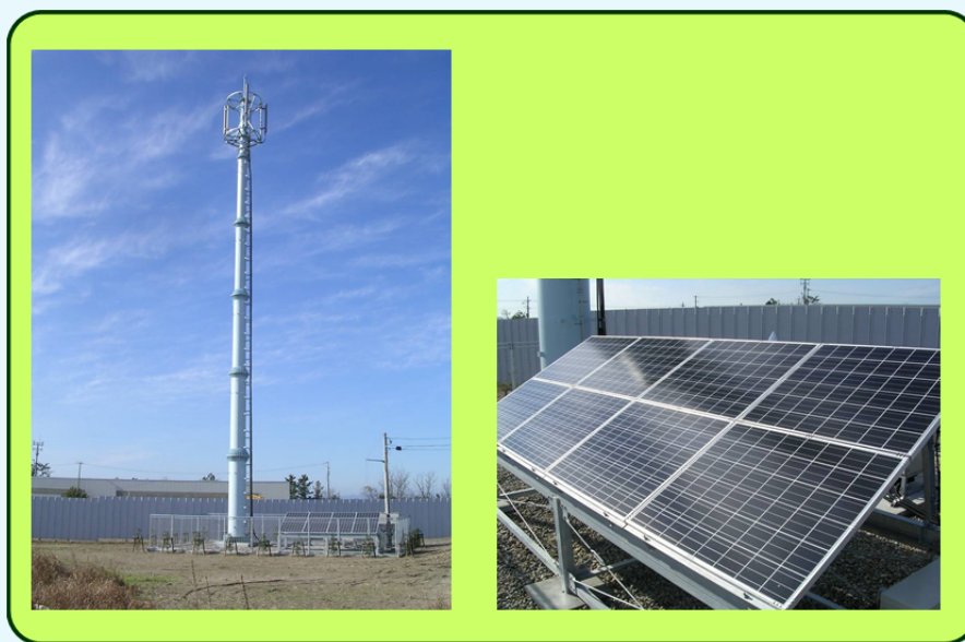
Figure 6.4 Equipment installed for tribrid technology field trials
