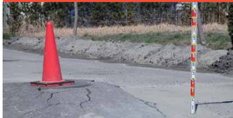
Photo 2 — Damage caused by subsidence
