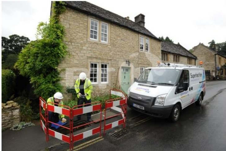
BT Openreach workers are taking 'Superfast Broadband' to rural areas of the UK. Image: BT
