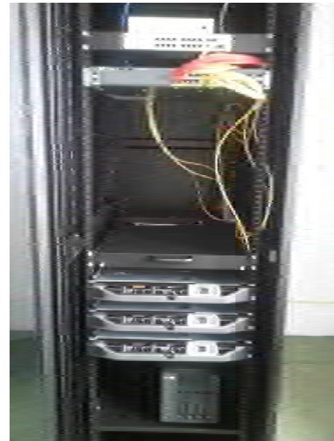
Municipal Server Installation
