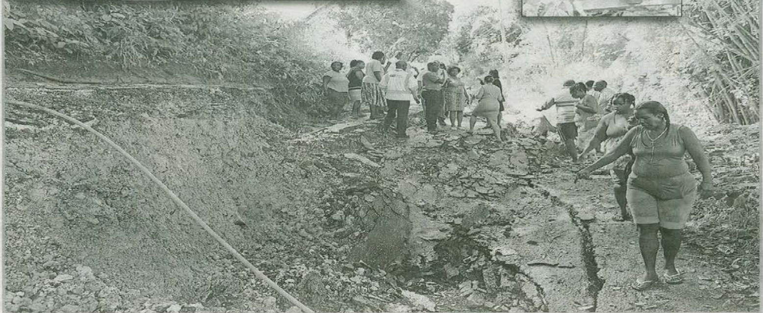
WHITE HILL RESIDENTS showing how much further the road collapsed on Tuesday night. Inset top left, officials from MTW at the collapsed road at White Hill.
