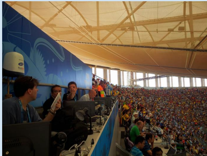
Figure 10: The new EMF monitoring system installed in Brazil's national stadium "Mané Garrincha" in Brasilia, during the 2014 FIFA World Cup
