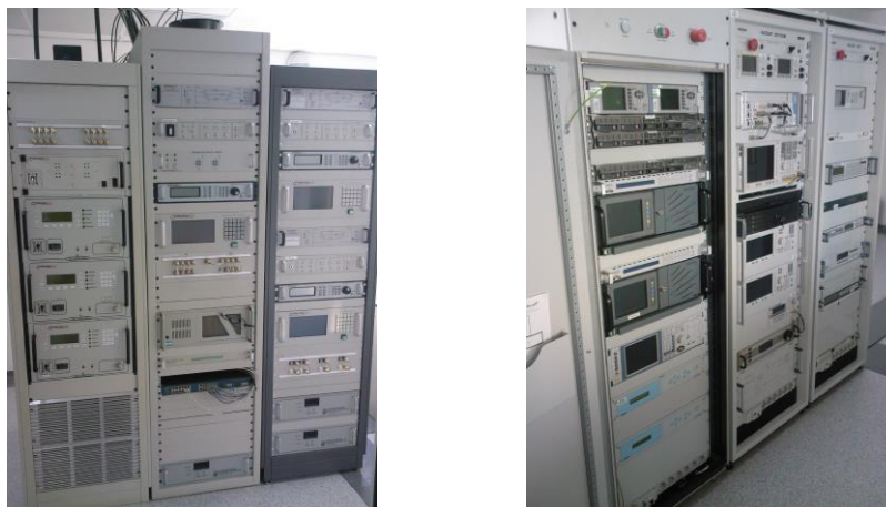
General view of the measurement equipment
