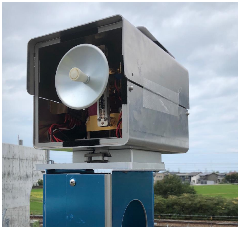
FIGURE 15 External view of trackside RAU
